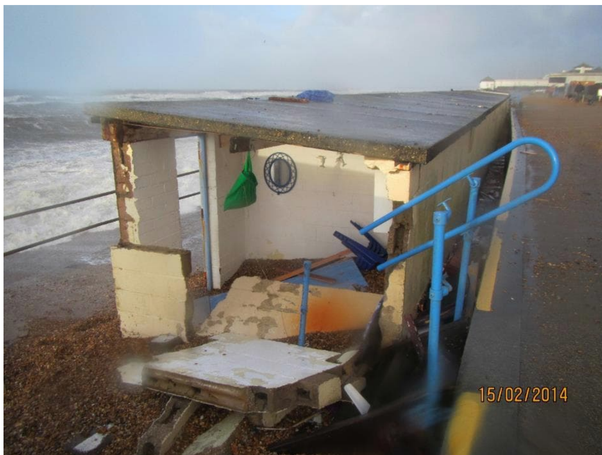
Figure 2-7: Photograph of damaged beach hut at Milford-on-Sea following February 2014 storm (obtained from NFDC)
